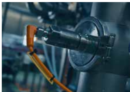
IO-Link sensors are utilised throughout the plant to provide real time performance data.
