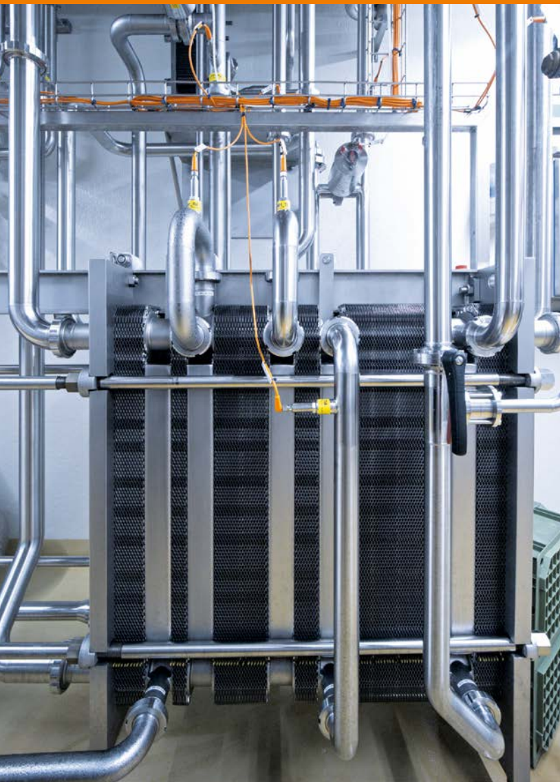
The heart of the plant: plate heat exchanger for accurate temperature control of the raw milk.
