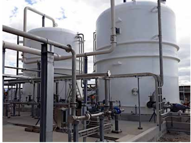
Te Maunga treatment plant
