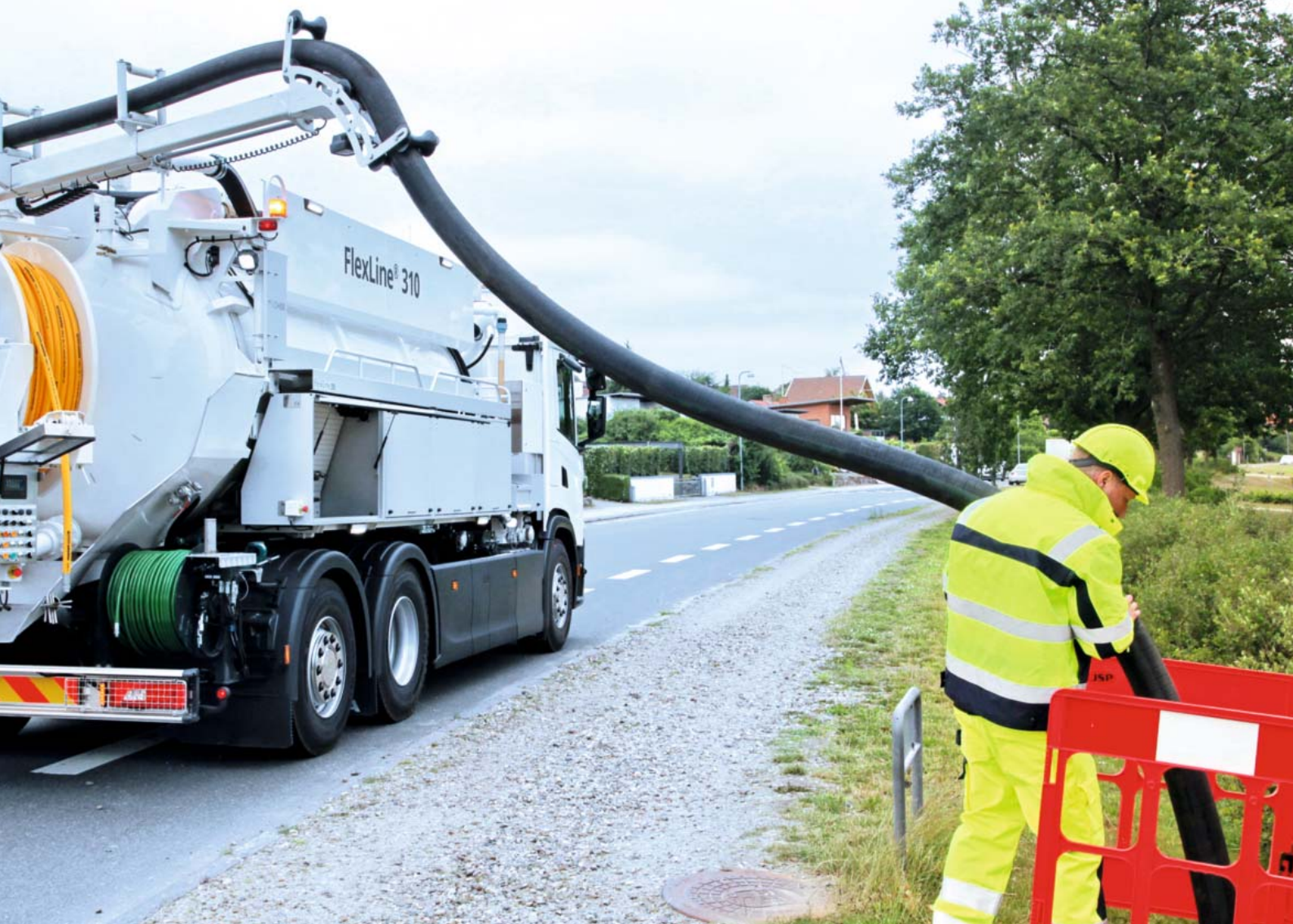
A sewer cleaning vehicle with the uncoiled jetting and suction pump for sewer cleaning.
