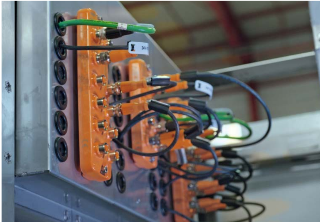
All sensors and actuators communicate with the controller via IO-Link modules.
