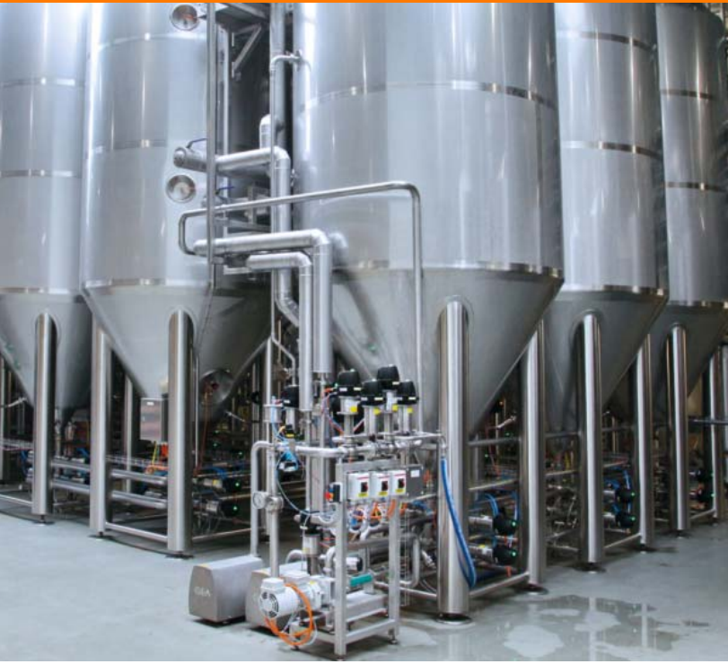
Numerous tanks are precisely monitored for level and temperature.
