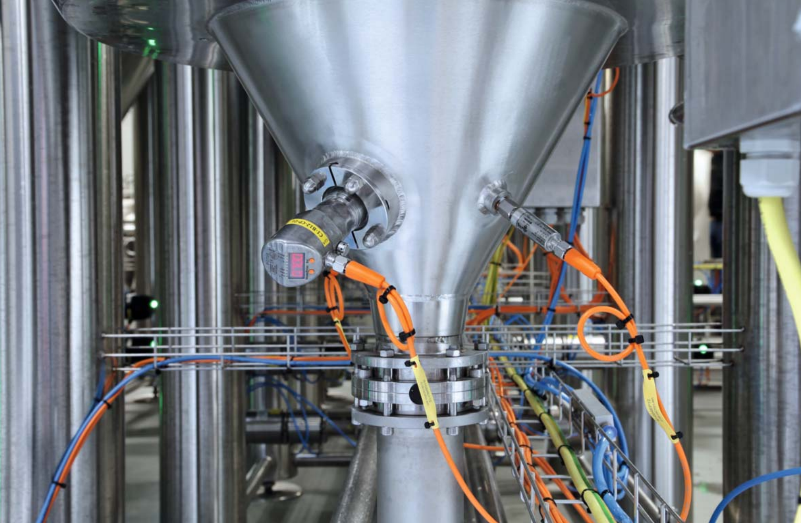
Pressure sensors for hydrostatic level detection (left) and temperature transmitters (right) are used to ensure a reliable brewing process.
