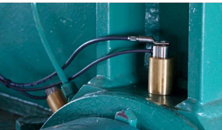
Two vibration sensors each, installed slightly shifted, permanently monitor the condition of the rotating bearings.
