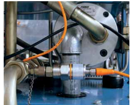
Long-term stable analogue values ensure reliable monitoring of hydraulic power packs.
