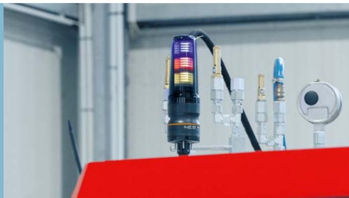
The IO-Link-based LED light tower is clearly visible from a distance and features an integrated buzzer.
