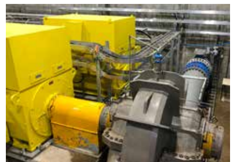
North Otago Irrigation pump station, employs ifm IO-Link condition monitoring systems. This state of the art pump station transfers 2 m 3 /s
