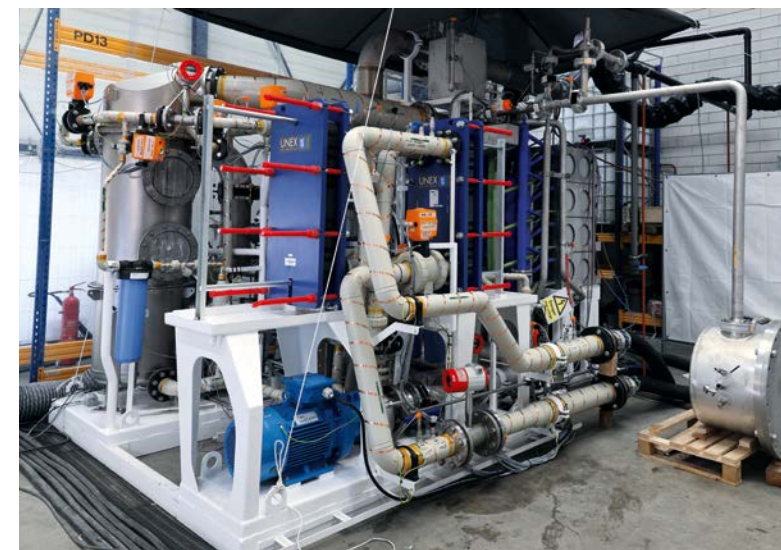
The K2 hydrogen generator developed by Koedood and Kooiman is tested before installation.
