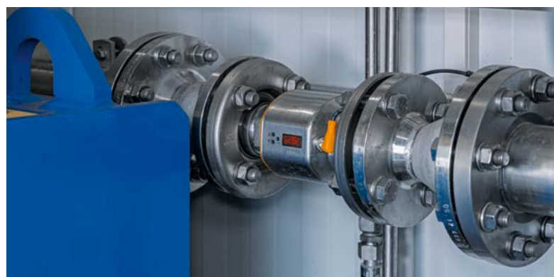
Central measured value: A magnetic-inductive flow sensor monitors the amount of sewage sludge entering the centrifuge.
