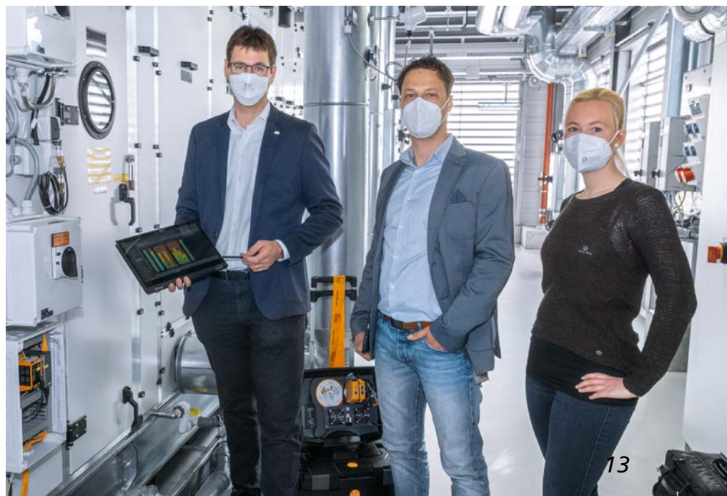
They have taken condition-based maintenance to a new level at the pharmaceutical company Boehringer Ingelheim (from left to right): Christian Ritz (Sales Engineer ifm), Rafael Cannas, Julia Kaufmann (both Specialist Maintenance Engineer at Boehringer Ingelheim)
