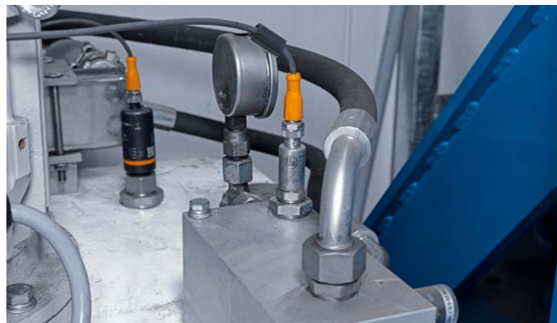
Monitoring of the hydraulic aggregate with regard to pressure, oil level and temperature.
