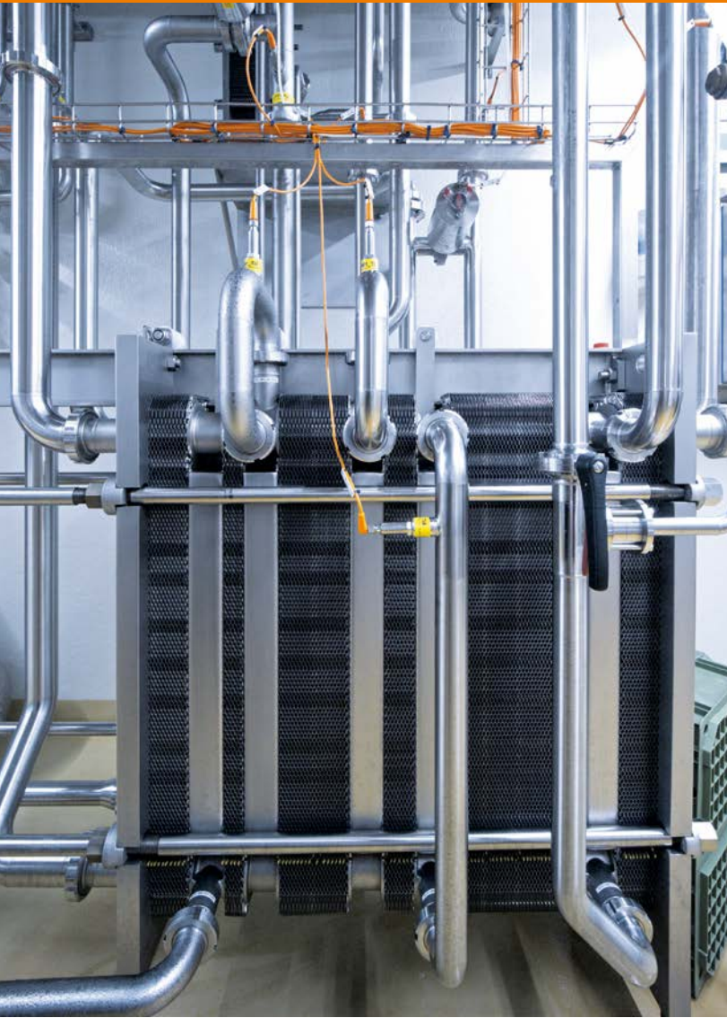
The heart of the plant: plate heat exchanger for accurate temperature control of the raw milk.
