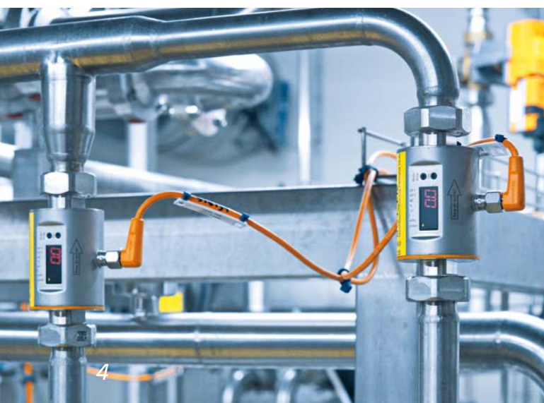
Magnetic inductive flow sensors in the permeate stage of the reverse osmosis system monitor and control the concentration of the whey.
