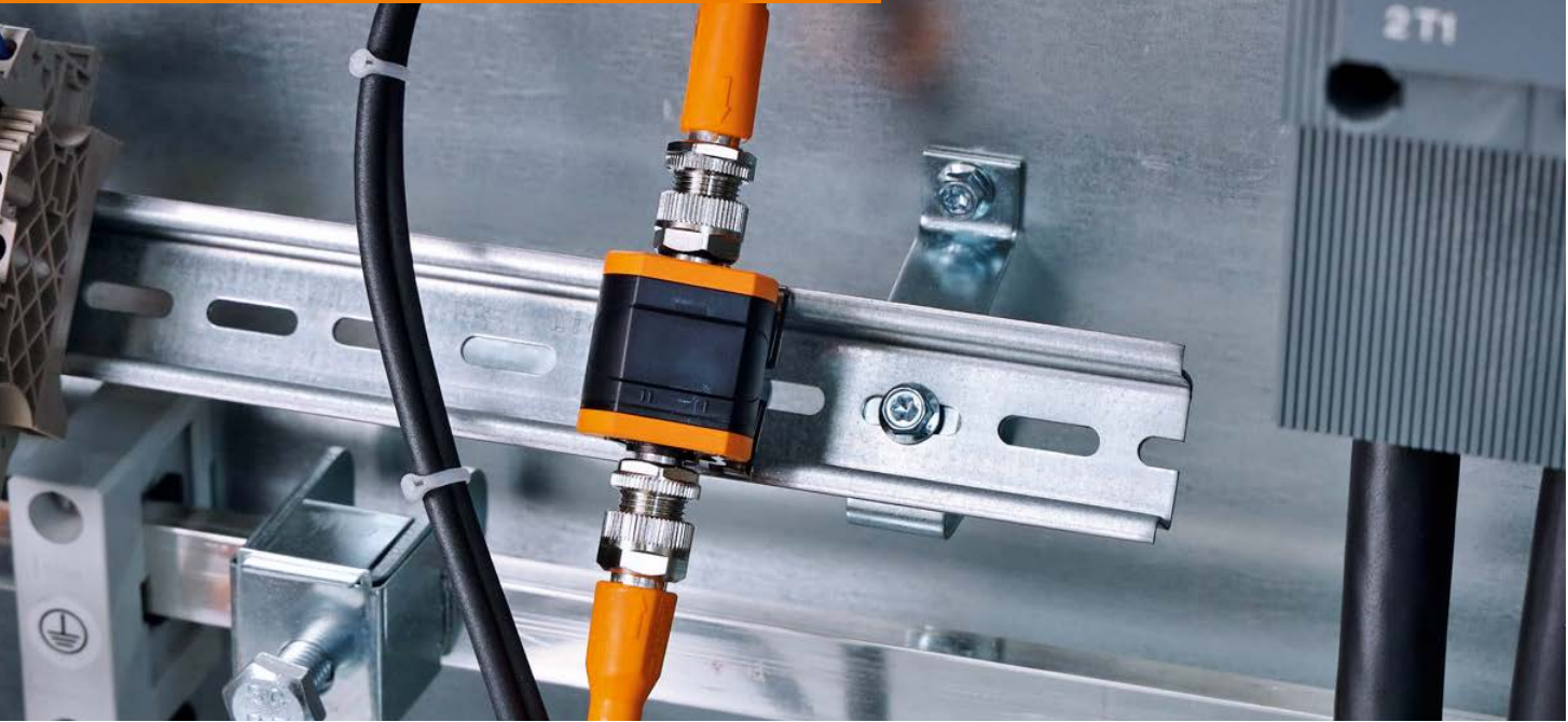
Even sensors without IO-Link can be integrated into the IT structure via data splitters.
