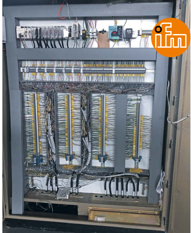
Before using IO-Link, two of these cabinets with analogue cards were needed to record the values of the sensors.
