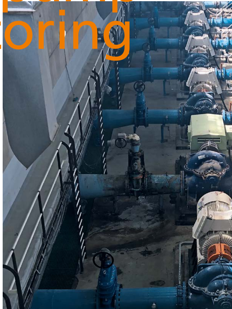
The high-lift pump station of Midvaal Water. The five newer motor-pump sets (grey motor housing) were equipped with IO-Link sensors and condition monitoring solutions.
