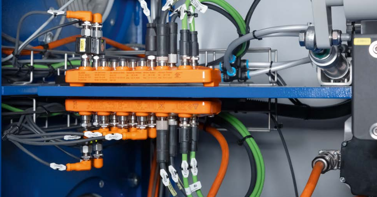
The signals from all the sensors are combined via IO-Link master and transferred to the machine controller via PROFINET.
