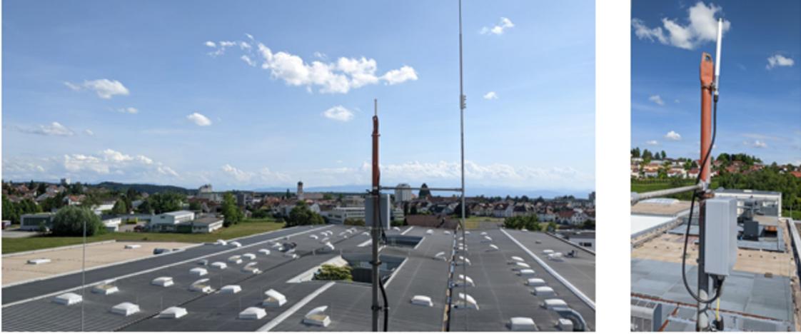
Figure 4: VIORITY BS mounted on the roof
