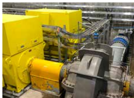
North Otago Irrigation pump station, employs ifm IO-Link condition monitoring systems. This state of the art pump station transfers 2 m 3 /s
